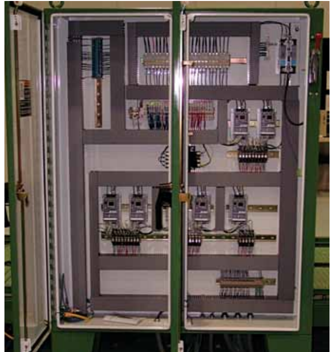
A Devicenet conveyor control system panel. The application was a distributed palette conveyor for warehousing. Photo courtesy of Connell Industries
